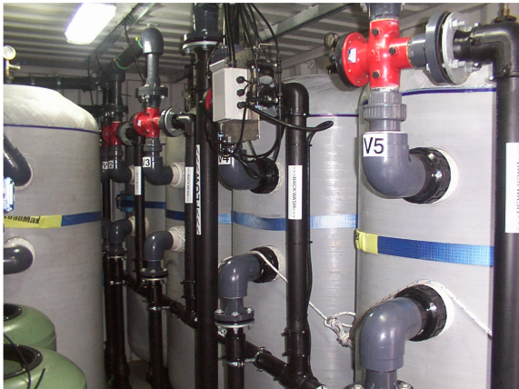
20' Sea Container Fitted with 50m 3 /hr Arsenic removal filtration system
