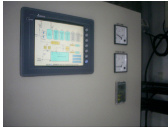
Touch Screen PLC Control system for Arsenic / Iron removal system
